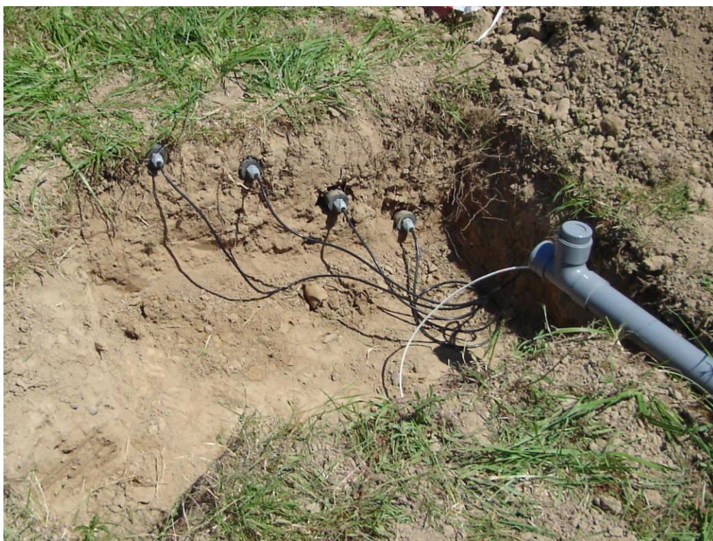
Figure S1.6 - Installation of the probes at Montaut (MNT).
