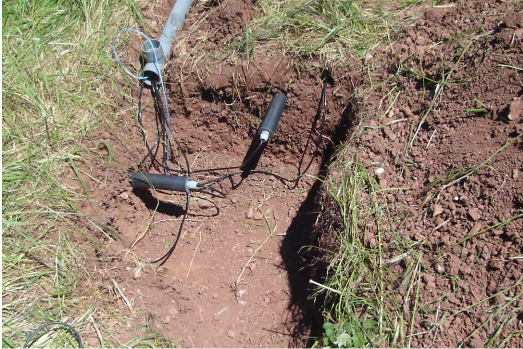
Figure S1.8 - Installation of the probes at Mouthoumet (MTM).
